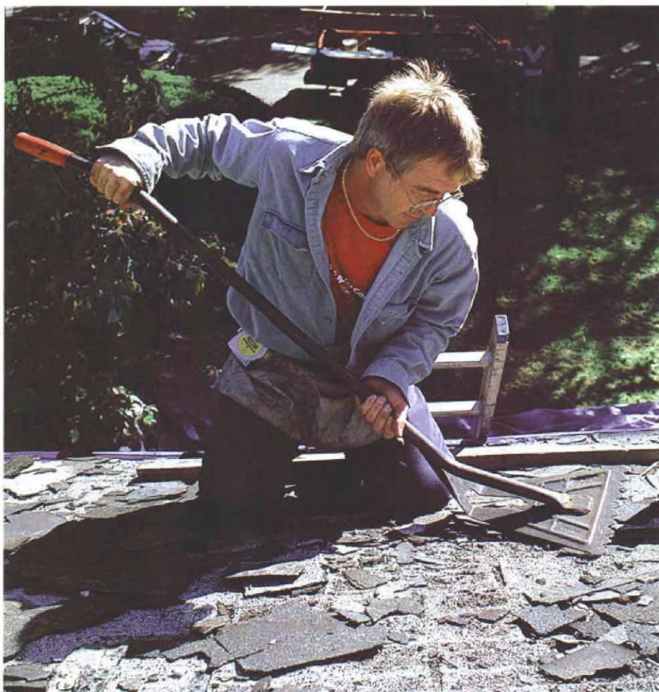
A roofer and a ripper. The main tool for removing shingles from the roof is a shingle ripper, or ripping shovel. Its flat, serrated blade gets under shingles and around roofing nails. The handle is angled steeply so that when you push down on it, you loosen both the shingles and the nails.
