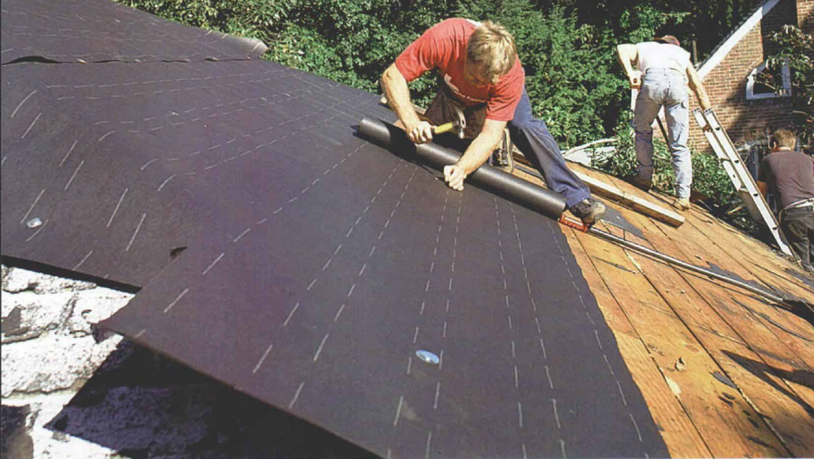
Roll out the paper. You can save a little extra work and keep from walking on the tar paper by papering from the peak down. Before nailing the bottom edge, tuck the lower course under the upper and fasten the whole shebang with roofing nails and tins, which hold the paper better than staples do.
