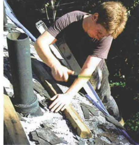
Spiking the cleat. A low-tech but effective foothold when working on a particularly steep roof is a 2x4 cleat spiked over the old roofing with 12d duplex nails, which are easy to pull out. These 2x4 cleats are spiked into the roof vertically every few feet, and a row of them continues unbroken across the roof.
