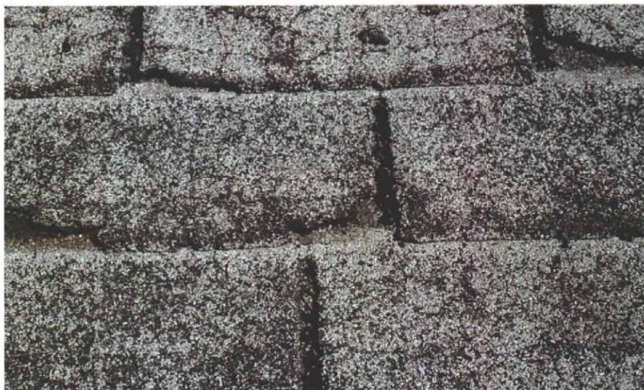
Past their prime. These deteriorated asphalt shingles have missing corners, and roofing nails show. They also snap and crumble easily, and the black showing through indicates that the protective layer of granules has worn away, leaving the asphalt exposed to the sun's ultraviolet rays.
