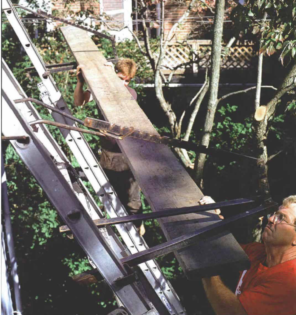
Setting up ladder brackets. With extension ladders tied off at the fascia, ladder brackets are hooked onto the ladders about 5 ft. below the eaves. Scaffolding planks—not framing lumber, which is too springy—span the brackets to give you a place to work from when you begin roofing.
